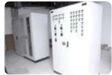
Signalling Indoor Equipment Installation at Sant Tukaram Nagar (STG) Station
