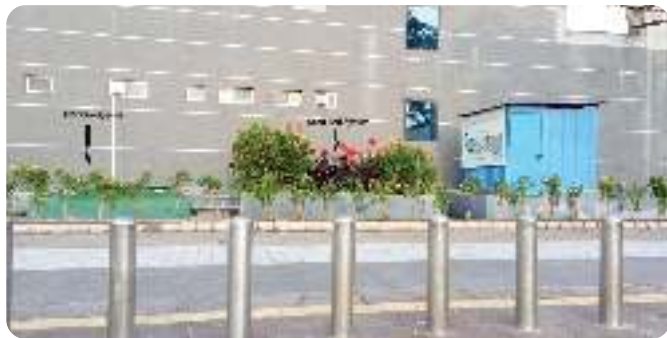
Actual Picture of Working STP at Airport South Station
