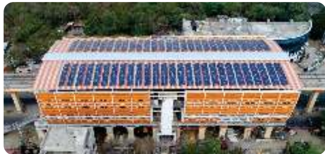
172.8 kWp Solar PV system installed at Airport Metro Station
